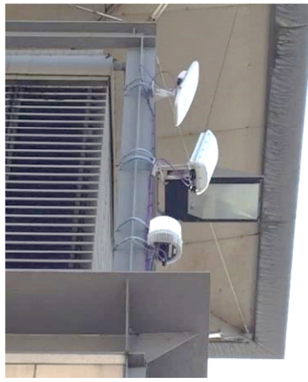
Figure 4: Wi-Fi APs in Millennium Square
